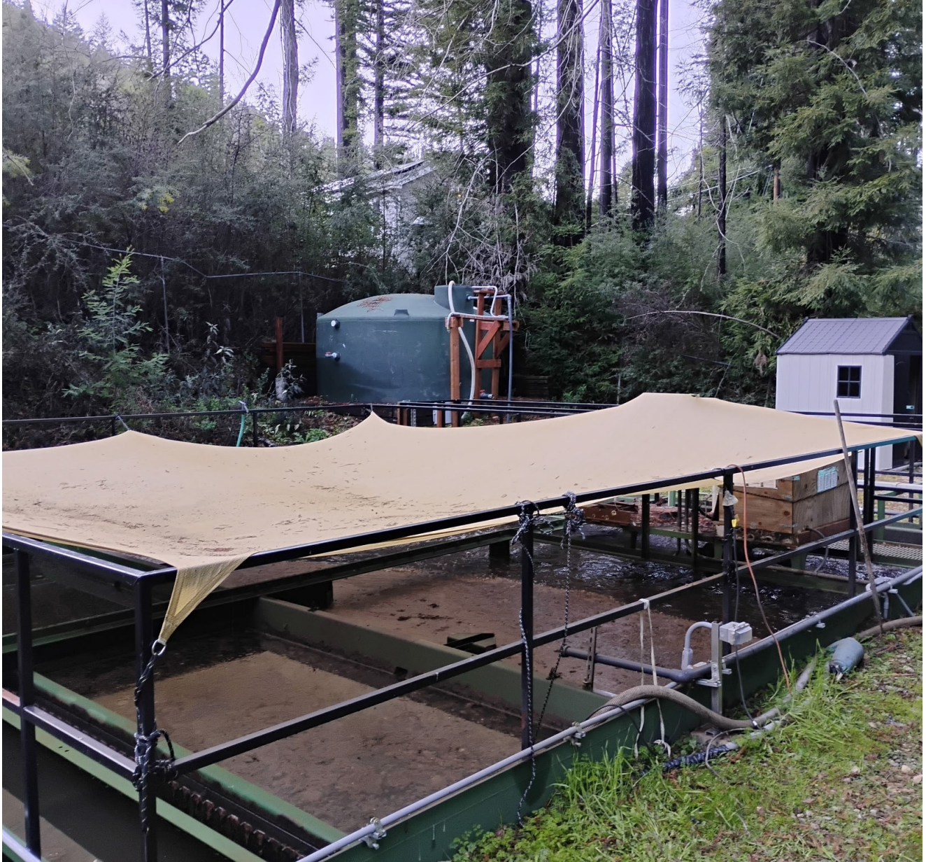
CSA 7 - Boulder Creek Zone 2 Big Basin Wastewater Treatment Plant
